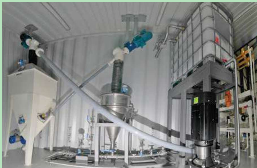
Water treatment system inside an ISO container
