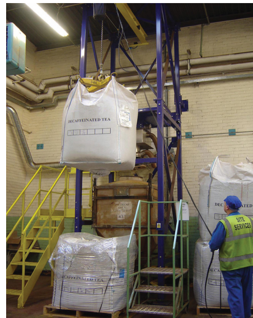
Hoisting bulk bag into the Discharger
