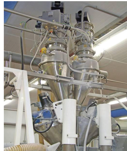
The vacuum transfer system to the packing machines
