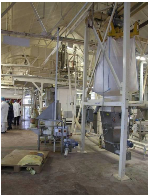
General view of the installation
