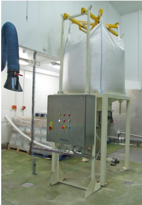
Bulk Bag Discharger with Flexible Screw Conveyor leading off through warehouse wall
