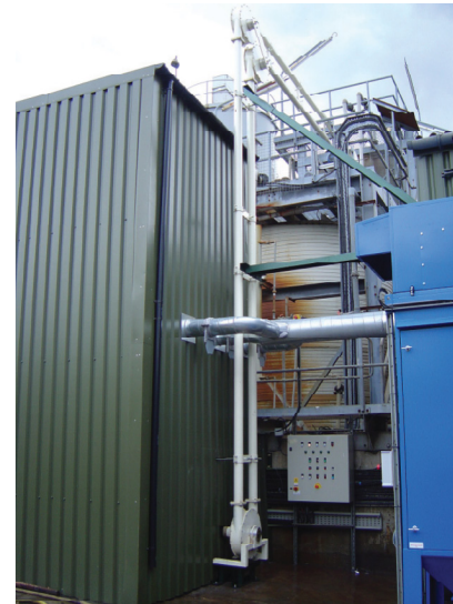
Spiroflow Aero Mechanical Conveyor transfers product from the Bulk Bag Discharger to a very large mixing Tank
