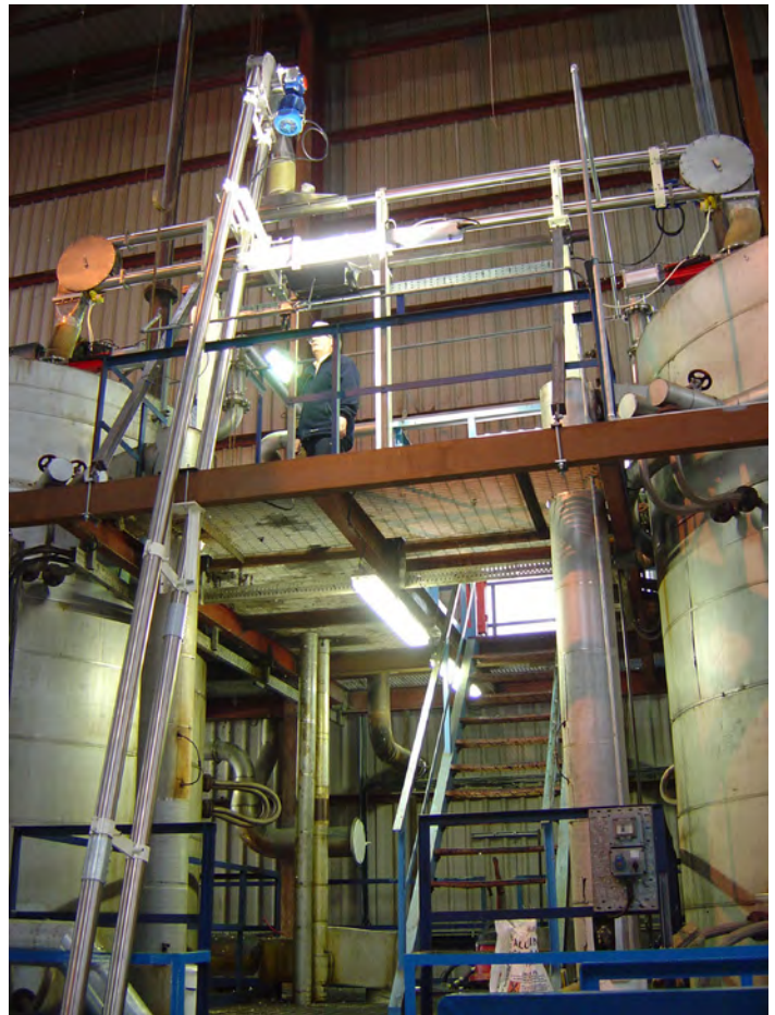
An Aero-Mechanical Conveyor (AMC) from Spiroflow Systems, Inc., Charlotte, North Carolina that operates high up into the roof area. In this situation, rope tension maintenance could be more difficult without the use of scaffolding or a mobile access platform.
