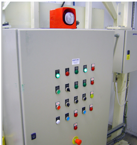
Control Panel designed in-house
