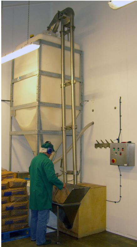
The Aero Mechanical Conveyor delivers sugar more quickly into the mixer.
