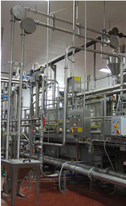
General View of the Aero Mechanical Conveyor installation
