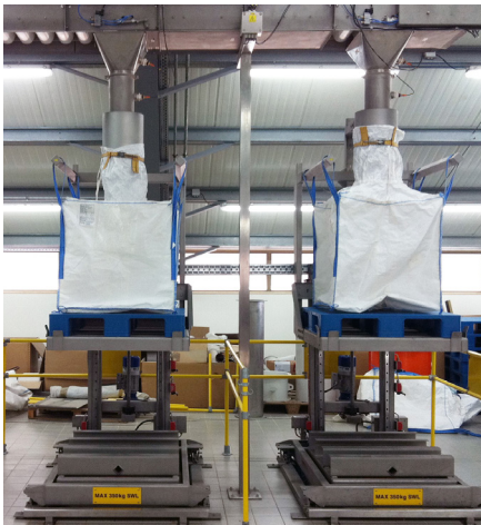
The bulk bag fillers in the 'rise' position
