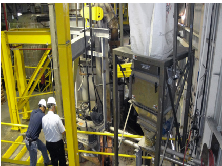
Spiroflow's Bulk Bag Discharger delivers hexamine powder into the Dynaflow chain drag conveyor at Hexion's Acme, NC plant.
