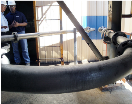
Acme Engineering Leader, David Swart, P.E. and Hexamine Production Leader, Joel Johnson, observing the back side of the Dynaflow chain drag conveyor installed through the building's exterior wall.
