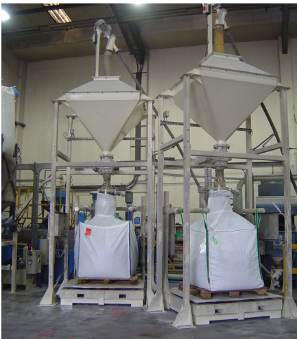
Flexible Screw Conveyors leading from the Rigid Bin Dischargers on the compounding line
