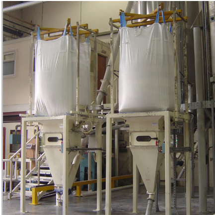
Bulk Bag Unloaders on pulverizing line
