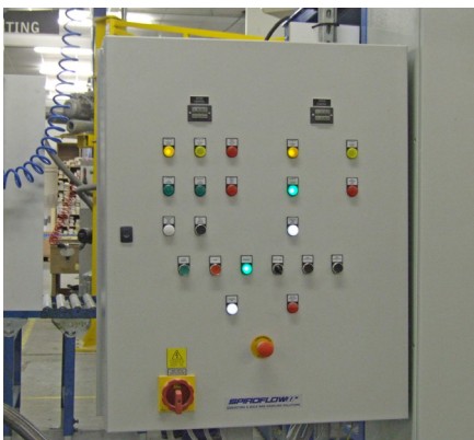
Main Control Panel
