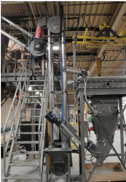
A vertical Aero Mechanical Conveyor moves cement powder from dual Flexible Screw Conveyors to a second Aero Mechanical Conveyor that extends through the building roof to an outdoor storage silo.
