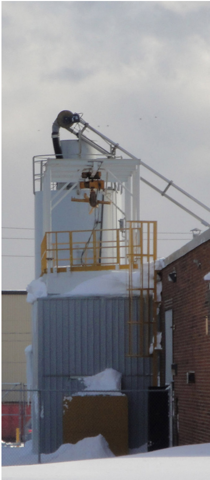
The Aero Mechanical Conveyor transfers material into an outdoor silo.
