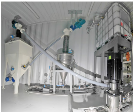
The 2 flexible screw conveyors inside the container
